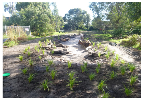
Photo of the newly built frog habitat connections beside the Sandringham Leisure Centre.
