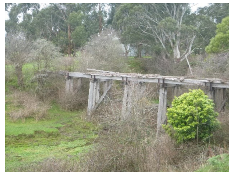
One of the existing trestle bridges along the Woolamai to Nyora rail trail that will need to be inspected in detail.
